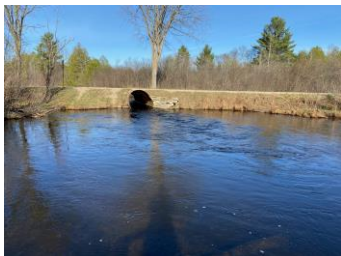
Deer Creek at Fuller Road is shown here with the culvert in place. —Photo taken on April 18.2021
