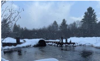
This is the calm before the culvert removal. —Photo taken Monday, December 2, 2024 at 9:54 am
