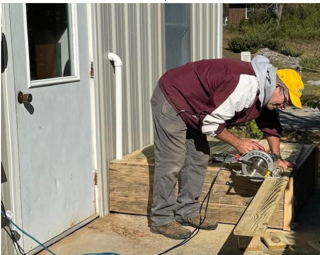
Volunteer Dave Clapp works on a bench that will serve a double purpose: to insulate water pipes and provide a place for visitors to sit a spell.
