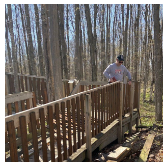
Volunteer, Dave Clapp, works to repair the railing along the treehouse ramp.
