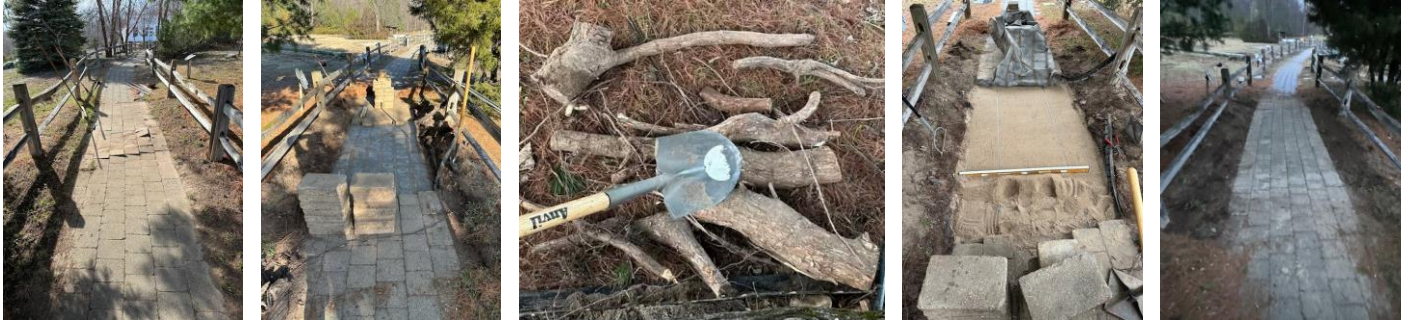
Tree roots were the perpetrators that buckled the Brussel blocks in the Permian section of Raven Hill's Exploring Beyond Jurassic Park walkway. Volunteer Jackson Brooks' attention to detail was meticulous as he removed the blocks, cut out the offending tree roots, then replaced the sand and Brussel blocks to make the walkway as good as new!
