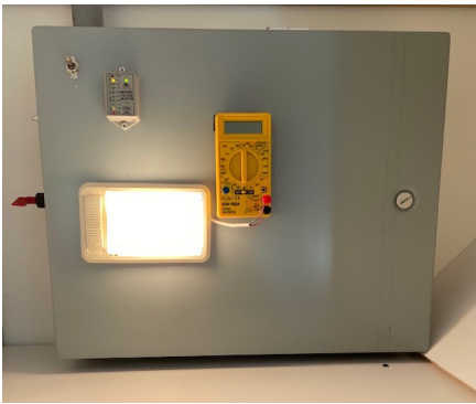
This light is wired directly to one of the solar panels. When a cloud goes over the solar panel, the light dims. When the sun comes back out, the light brightens again.
