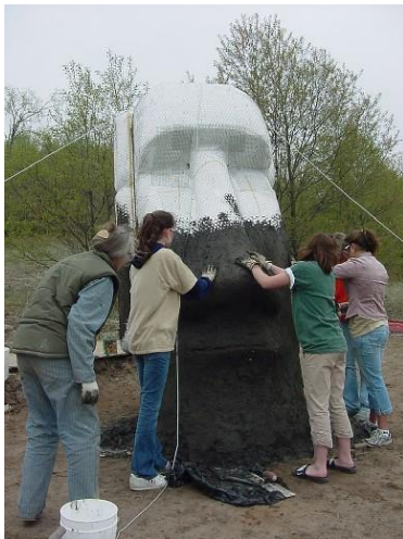
Getting down and dirty with the first coat of cement, middle girls learn some practical chemistry.
