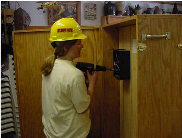
In 2003, a group of middle school girls from Charlevoix and Emmet County schools participated in a Raven Hill grant program called Work SMART . They learned the Science Math And Related Technologies (SMART) of Work. Their carpentry, electrical, plumbing & masonry work is still displayed at the Center on occasion.
