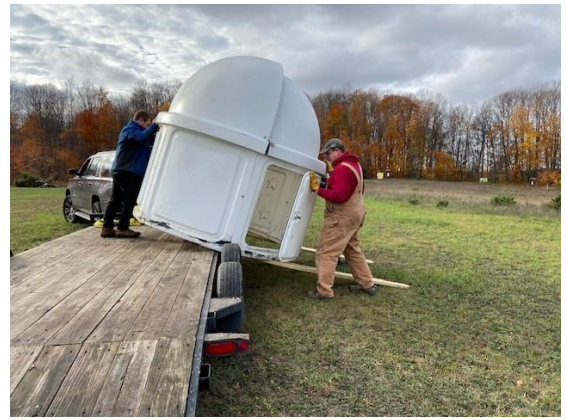
Never has a project gone so smoothly. The observatory slid off the trailer to its new location. Not only was the landing site perfectly level, there was not one single rock hit as rods were pounded into the ground to secure the dome.
