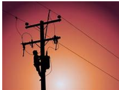
A lineman maintains electric power lines. This is a dangerous job, when the live wires come down.
