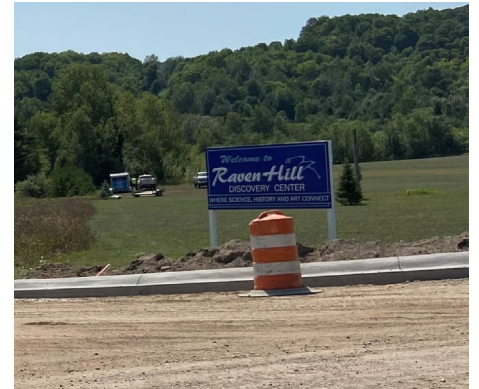
It has been a real experience just getting to Raven Hill this week! There is road construction on C-48, INCLUDING new curb & gutter at the intersection of Pearsall & Fuller Roads. Plus, the Charlevoix County Road Commission has been busy trimming the trees along Fuller Road. Thanks to everyone involved in all these upgrades.
