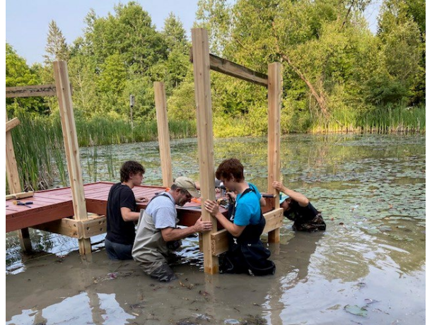
Eagle Scout Dylan Clapp and his crew stayed cool in the water, as they worked on the new dock system they are installing at Raven Hill's pond.
