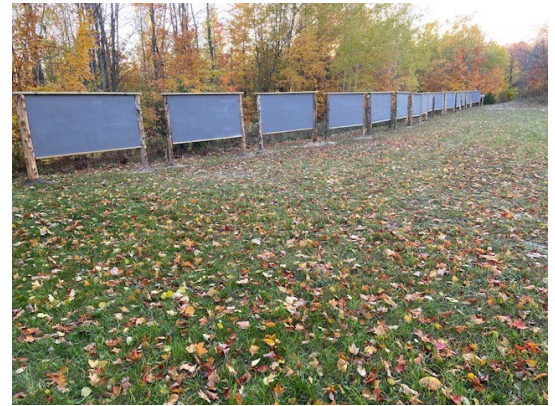
In October, the 8' x 4' panels were constructed to create a timeline of technology from Stone Age to Modern. Now they patiently wait for the actual exhibit to be installed. The panels already guide visitors to the Wetlands Boardwalk and the Ancient World.
